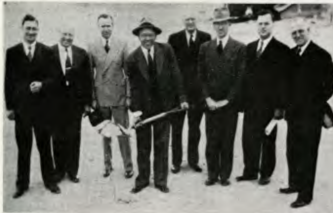
J. W. Turner, president of the Southwestern Union Conference, turned the first shovel of dirt during the ground-breaking ceremonies on April 14, 1947, for the school's administration building.
