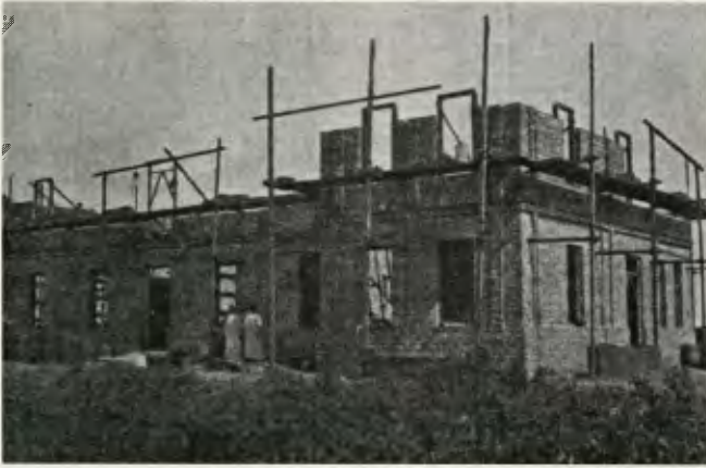
Construction of the sanitarium at Entre Rios continued only as quickly as funds were received to purchase the necessary materials.
